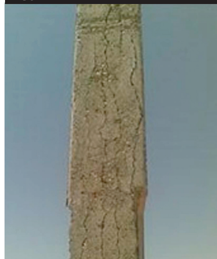
The concrete cover on this power pole cracked and fell off as a result of high-voltage AC leakage.
